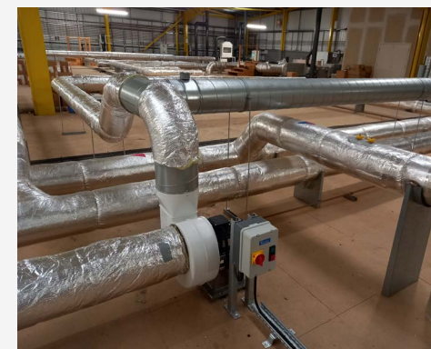
Wakefield, UK, Redirected ducting
